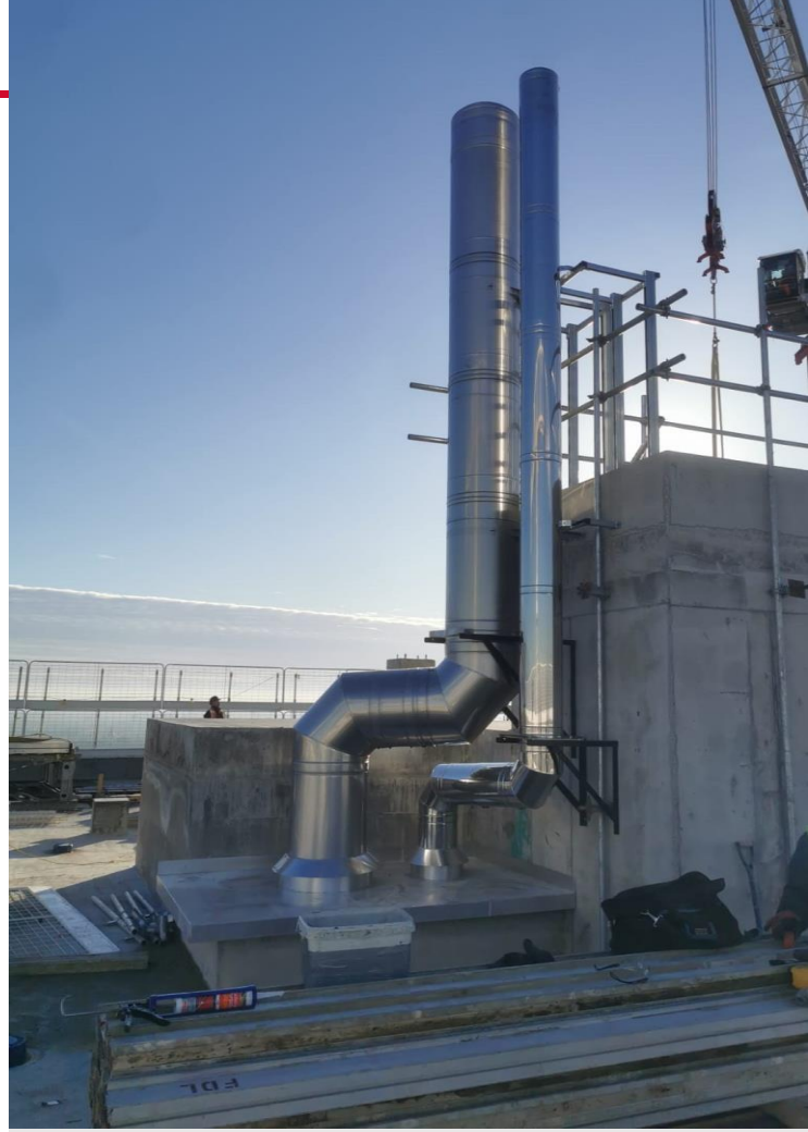
Our Boiler and CHP flue systems installed above roof level.
