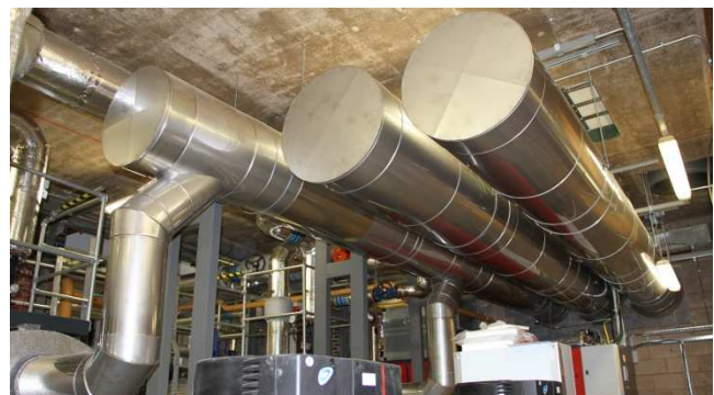
Flue systems within the plantroom
