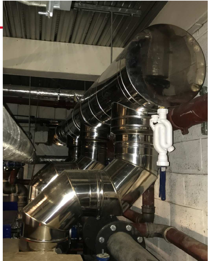
Flue header system within the plantroom
